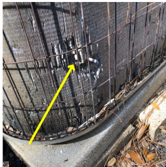
Corrosion and damage on condensing unit.
