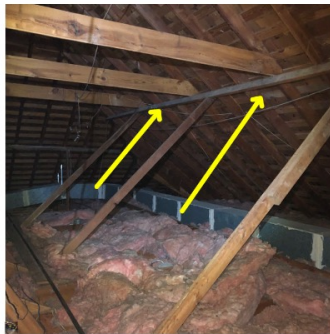
Missing purlin brace(s).
