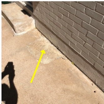
Patched concrete, Exterior Right.
