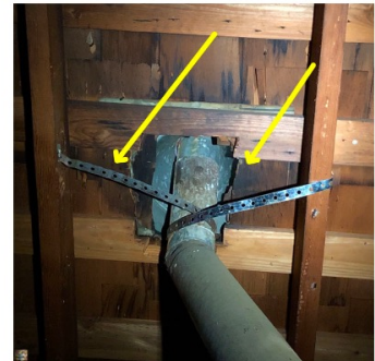
Stains on underside of roofing.
