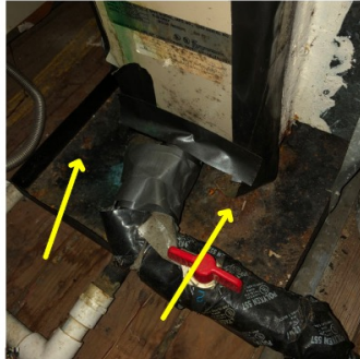
Corrosion and/or debris in the condensate drain pan.
