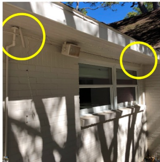
Condensate line terminations.
