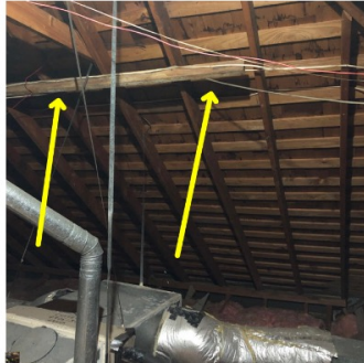
Missing purlin brace(s).
