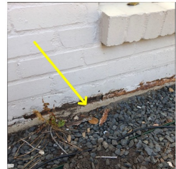
Damaged foundation or slab. Exterior Rear
