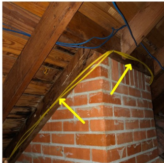
Wood framing improperly in contact with chimney.
