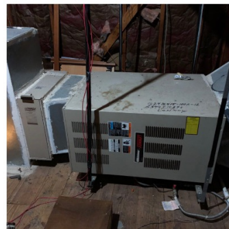
Furnace location(s): Attic
