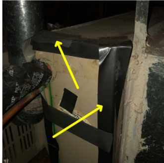
Improper tape on evaporator and refrigerant line.
