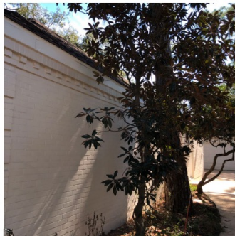
Tree in close proximity to foundation.
