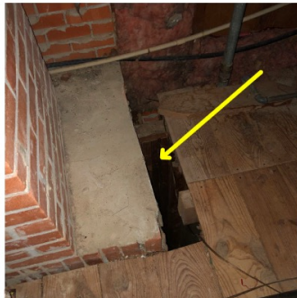
Opening not firestopped or insulated. Attic.
