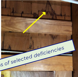
Stains on underside of roofing.
