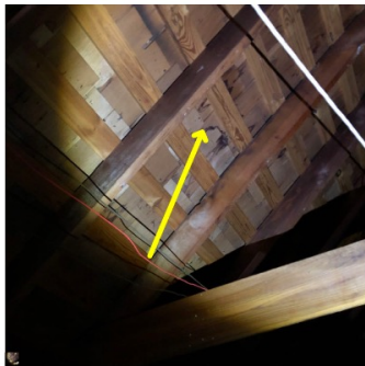
Stains on underside of roofing.
